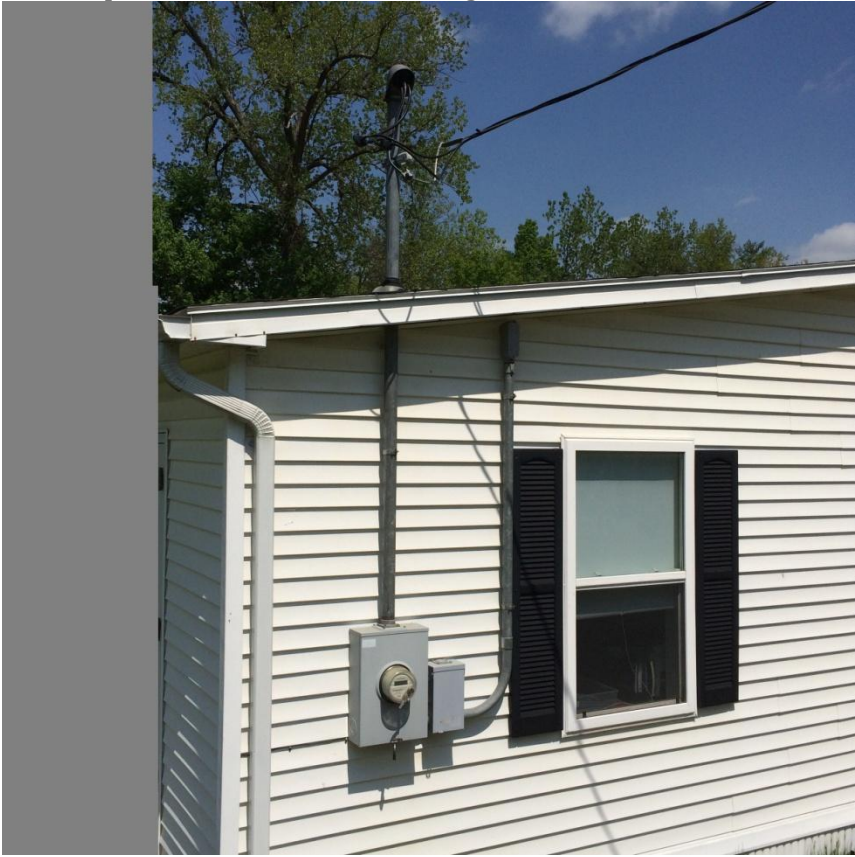
100 amp service on side of existing unit on Mohawk Trail side
